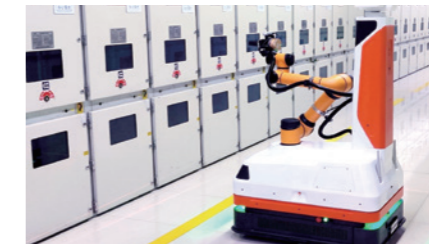
High-voltage distribution cabinet operation
